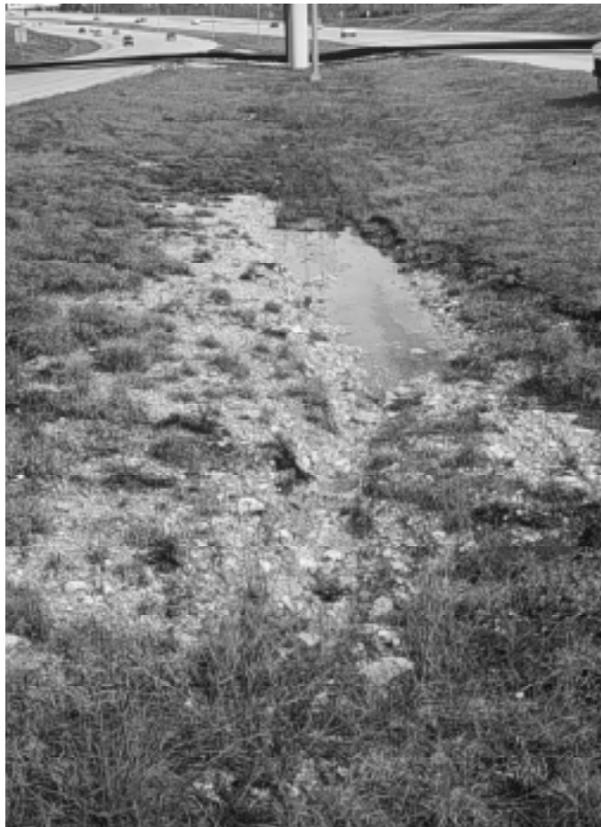
Figure 4.7. Erosion at the Walnut Creek vegetated buffer strip.
